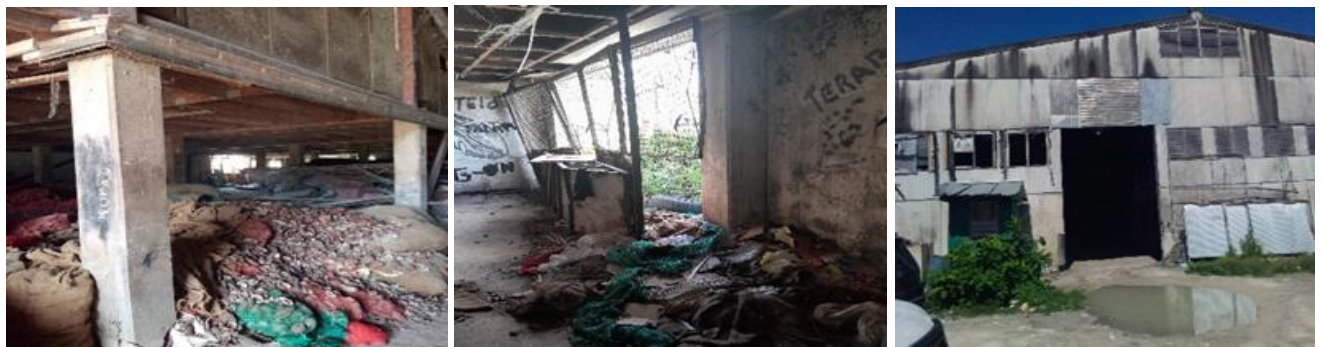
Figure 5 Examples of insecure and poorly maintained copra sheds
